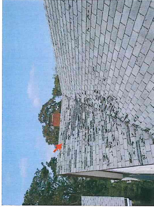
EXISTING ROOF - MAIN HOUSE SHOWING DETERIORATION
