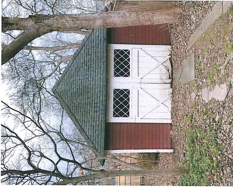
EXISTING ROOF - GARAGE SHOWING WEAR (MOSS GROWTH)
